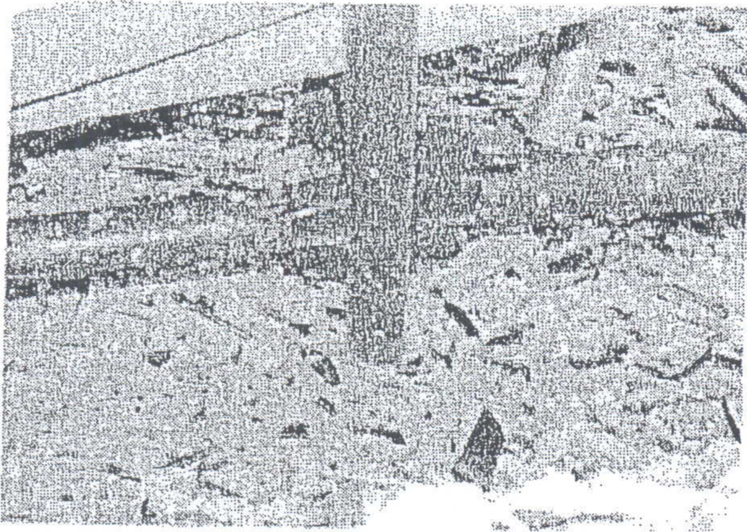
Pic. 19 Typical base of collapsed scaffolding. Note lack of base plates.
